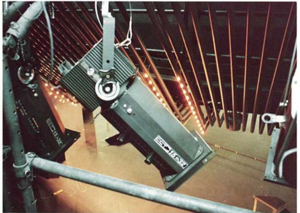
One of the CCT Silhouettes, part of the comprehensive lighting and effects package at the theatre.
